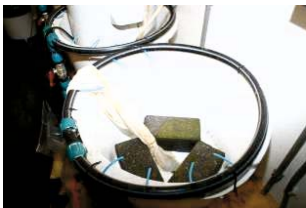
Installed cooling system
