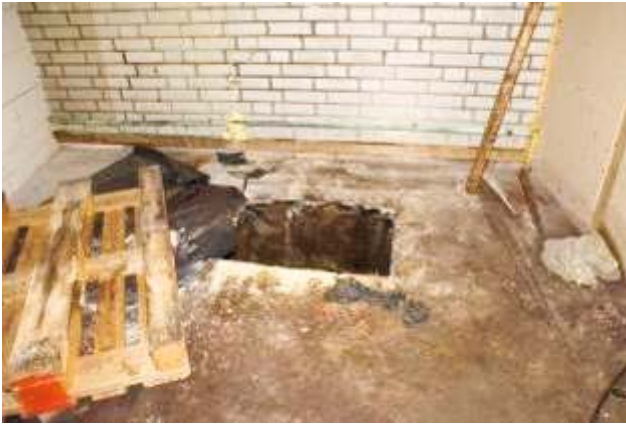
Hole hacked in the floor
