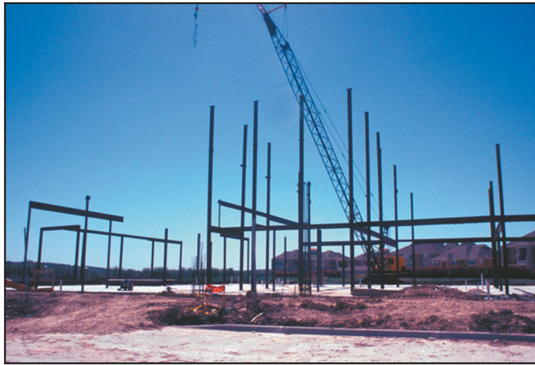
FIGURE 19.16 The erection of a steel frame begins with the erection of columns. The columns, with their shop-welded base plates, are anchored to the bolts embedded in the foundations (see Figures 19.18 and 19.19) by the general contractor as per the fabricator's details. In a multistory building, each column shaft is generally two stories tall.
