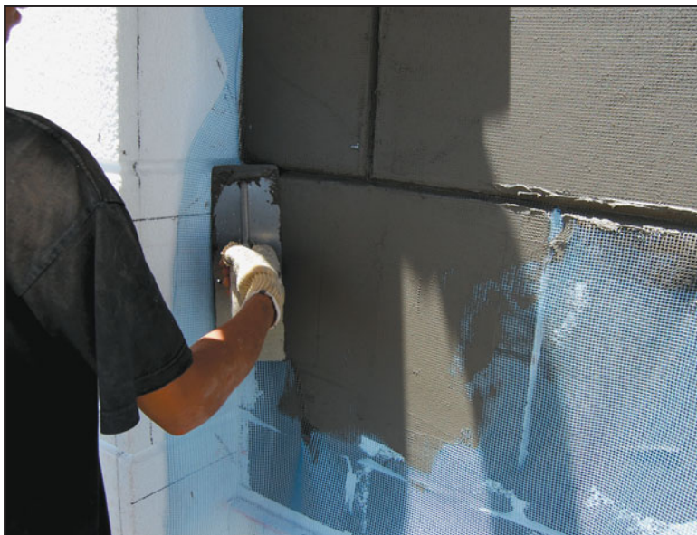
FIGURE 29.26 In applying the base coat, the base coat adhesive is first troweled on the insulation. Then the mesh is unrolled over the adhesive and an additional layer of base coat adhesive is applied. This embeds the mesh fully in the base coat.
