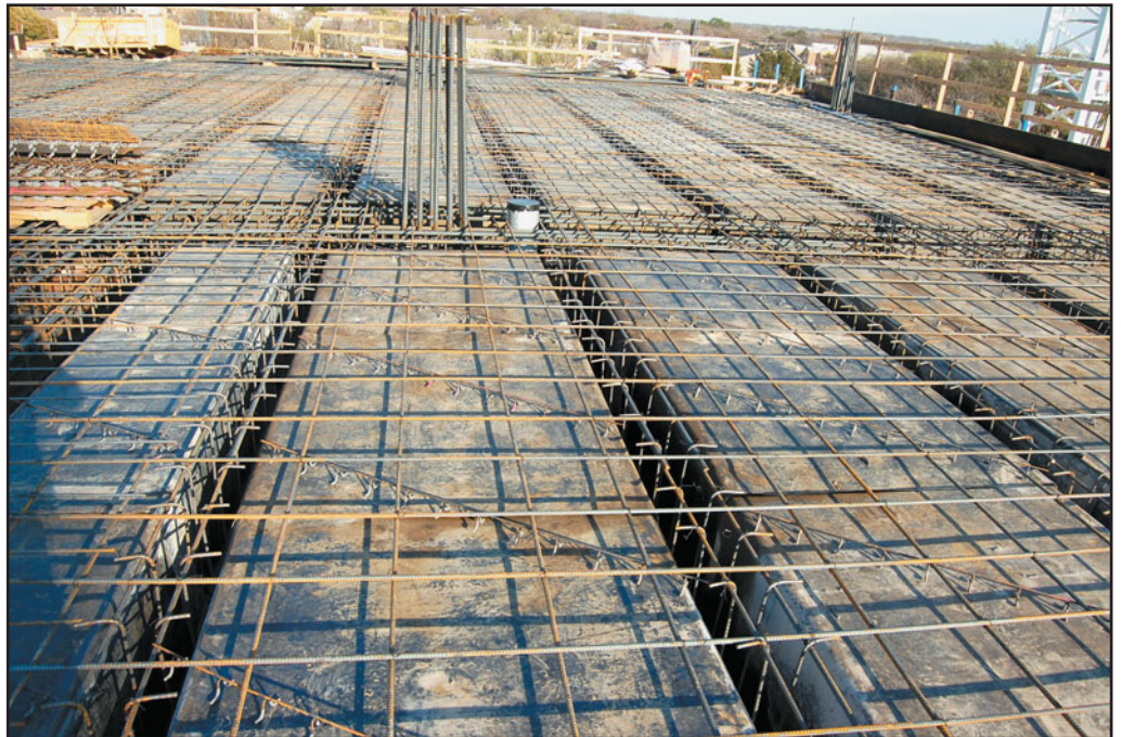
FIGURE 23.11 An overall view of a wide-module one-way joist floor formwork with rebars in place—ready to receive concrete. Observe the use of shear reinforcement (stirrups) in the joists.
