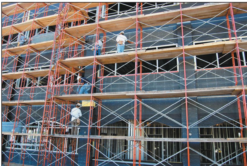
FIGURE 29.4 A five-story building facade covered with scaffolding for the application of stucco.
