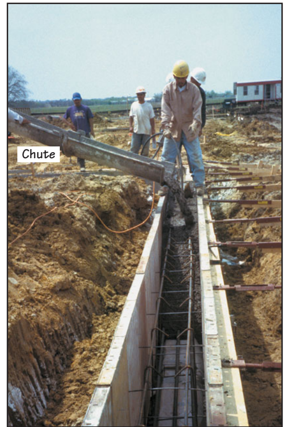
FIGURE 21.24 Concrete being brought into the formwork of a grade beam through an open chute from the mixer.
