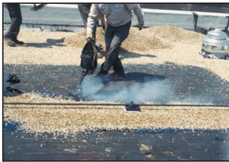
FIGURE 33.3(d) The bitumen under aggregate surfacing is poured over the deck, not mopped. That is why it is called a flood coat of bitumen.
