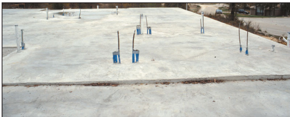
FIGURE 2 A typical completed slab-on-grade ready to receive the WLF superstructure. Note that the utilities extend above the slab (referred to as stubbed out of the slab).
