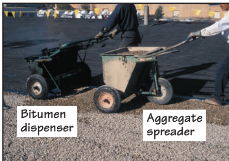
FIGURE 33.3(f) Although the bitumen for a flood coat can be poured with buckets, as shown previously, it is usually poured on large roofs using a bitumen dispenser followed by an aggregate spreader.
