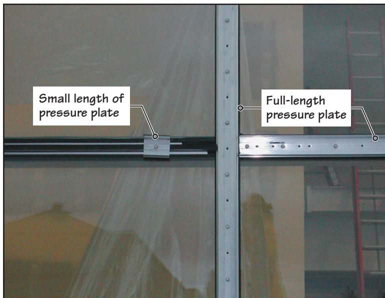
FIGURE 32.7 (b) In fastening the pressure plates to curtain wall framing members, the glass is temporarily held by small pressure plate members. After several glass panes are in position, the temporary pressure plates are removed and replaced by full-length pressure plates.
