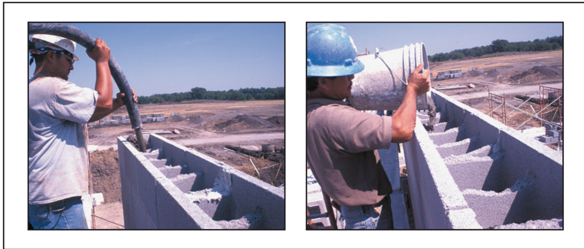
FIGURE 25.26 Two alternative methods of placing grout are pumping and bucketing. In these images, the masons are placing the grout in the cells of underlying CMUs. The CMUs showing at the top of the wall are bond beam units, which will be provided with horizontal reinforcement at a later date.
