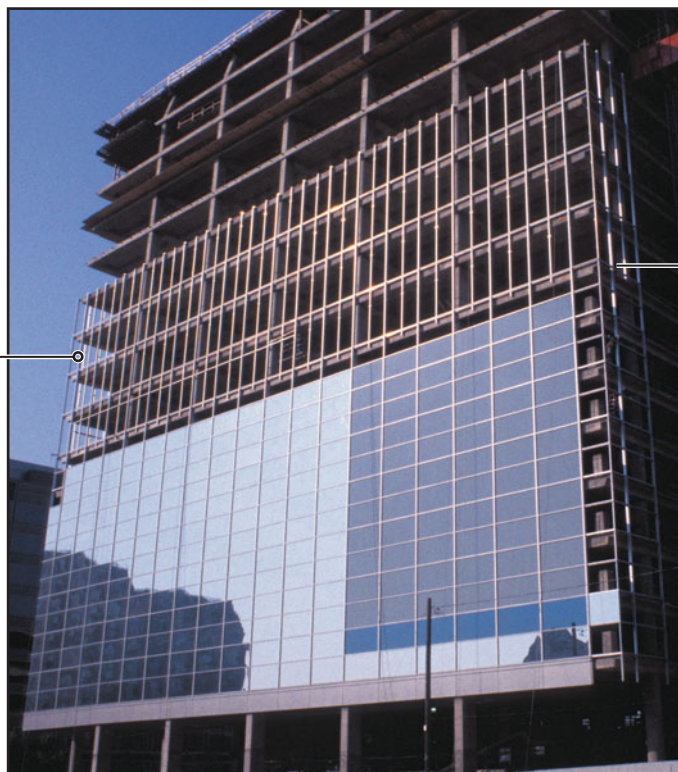
FIGURE 32.2 (b) The progress in the installation of a stick-built glass curtain wall on an office building in which the lower floors are parking floors and the upper floors are office floors; see also Figure 32.2(a).
