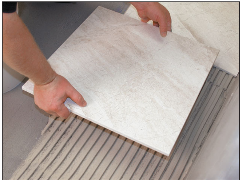
FIGURE 36.6 A closer view of setting large-format tile in mortar. The purpose of the notched trowel is that when the tile is set and pushed into place, the mortar will redistribute itself into a uniform bed. (Photo courtesy of Mapei Corp.)
