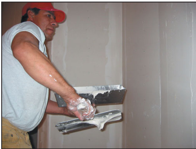
FIGURE 16.22 A drywall worker uses a pan containing the joint compound (mud) and a knife to apply it. (Photo courtesy of Tommy Eaton)
