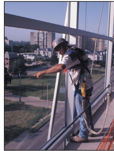
FIGURE 32.12 In an inside-glazed curtain wall, the covers are installed before the glass. In this photo, an installer is installing the snap-on cover on the mullion from an upper floor, and is helped by an installer at the lower floor. In an outside-glazed curtain wall, the covers are generally installed after installation of the glass and pressure plates.
