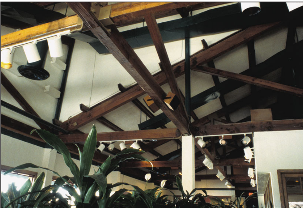
FIGURE 7.11 An example of heavy timber construction—Type IV. Notice heavy sections of wood with no protective covering and no concealed spaces.
