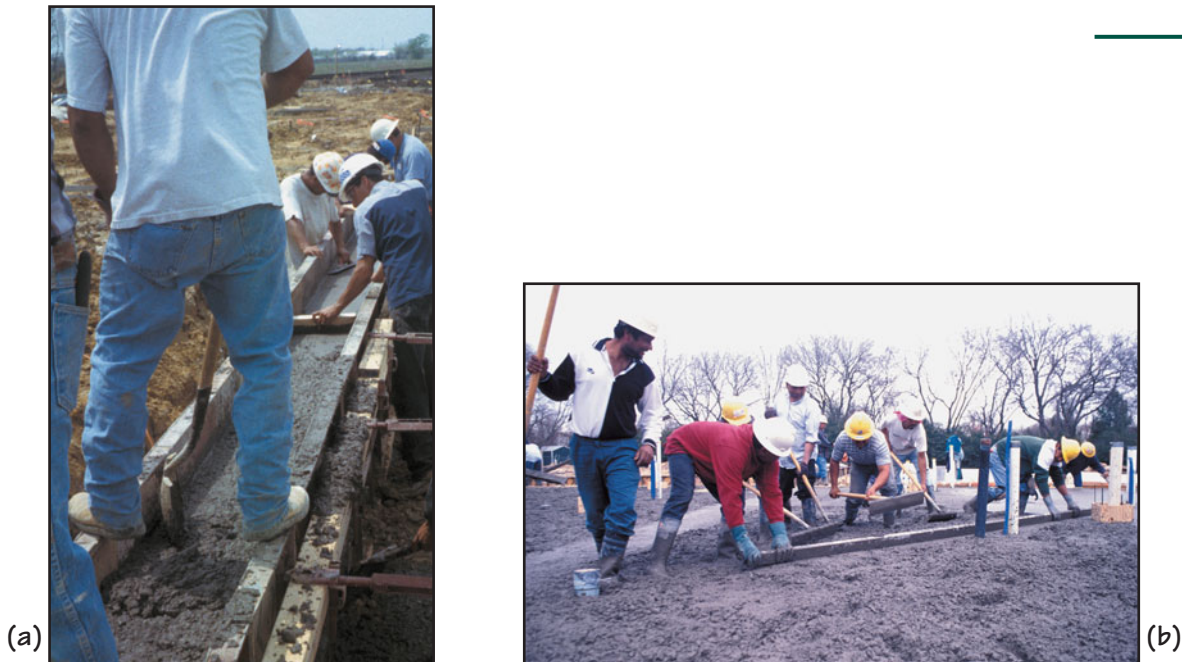
FIGURE 21.29 (a) Striking concrete in a beam with a wood straightedge. (b) Striking concrete in a slab with a wood straightedge.
