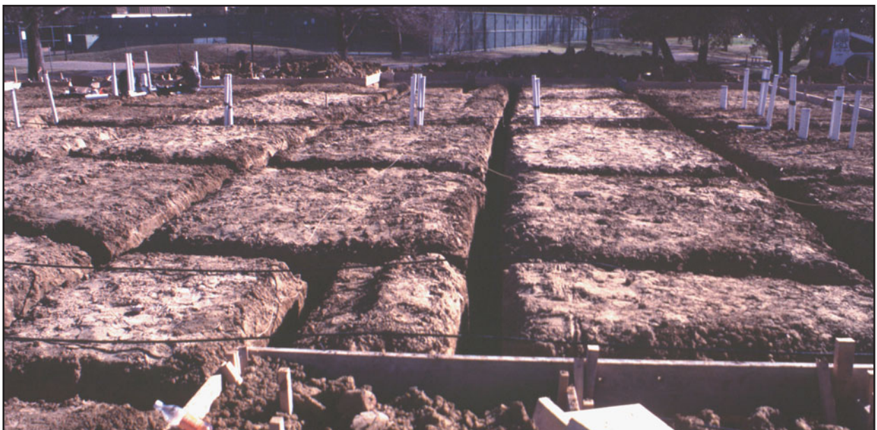
FIGURE 12.20 Excavation for a typical reinforced concrete slab-on-ground foundation showing the network of trenches in both directions. The trenches serve as formwork for concrete beams.
