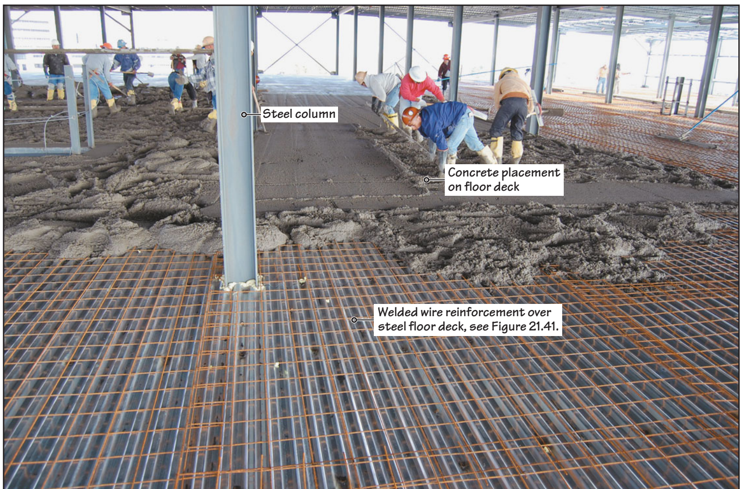
FIGURE 18.27 This illustration shows the placement of concrete on a floor deck (a form deck in this case). Observe the steel reinforcing bars placed over the deck.
