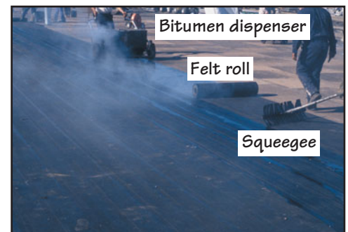
FIGURE 33.3(b) Although bitumen can be applied with mops, it is more convenient to use a bitumen dispenser on large roofs. The unrolling of felt over bitumen is followed by pressing the felt down with a squeegee.
