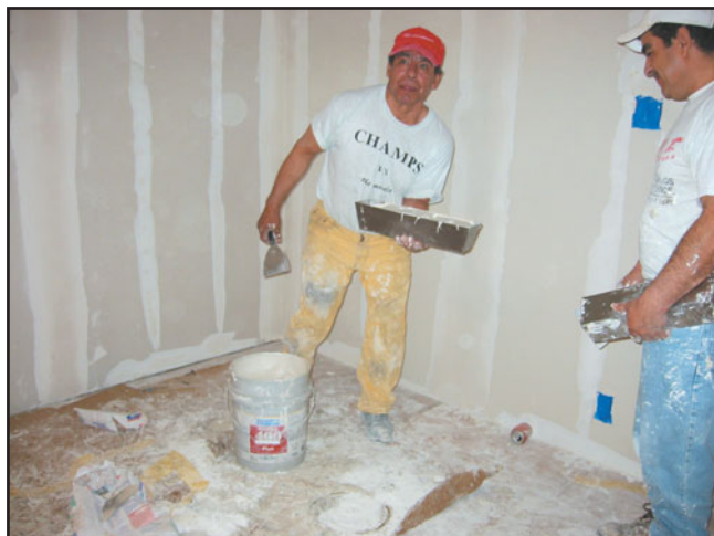
FIGURE 16.28 A room interior ready to receive paint. (Photo courtesy of Tommy Eaton)
