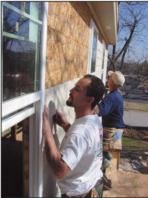
FIGURE 16.6 Installation of horizontal siding. Note that doors and windows are installed before siding is applied. In this building, an (outside) air retarder has not been installed because of the use of closed-cell, foamed-in-place insulation between stud cavities, which functions both as insulation and as air retarder; see Section 6.2.
