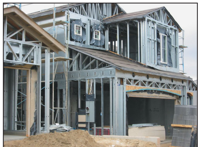
FIGURE 20.13 The exterior of a single-family dwelling in which all load-bearing and non-load-bearing walls, floors, and roof are framed with CFS members. Observe the similarity of framing of this building with that of a wood light-frame building. (Photo courtesy of Dietrich Metal Framing)
