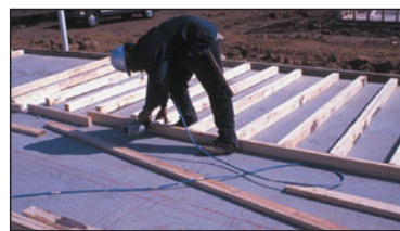
FIGURE 6 Walls are typically framed on the slab or floor platform and subsequently tilted up into position.
