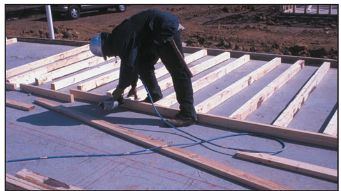
FIGURE 6 Walls are typically framed on the slab or floor platform and subsequently tilted up into position.
