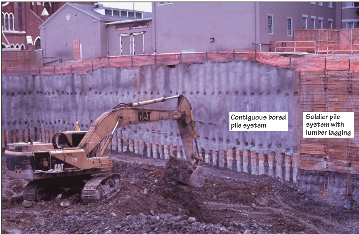
FIGURE 11.23 Contiguous bored piles used as supports for a deep basement excavation in a tight urban location. In areas farther away from the existing building or property line, the soldier pile and lagging system is used. Note that as the excavation proceeds, the lower part of drilled concrete piles will also be shotcreted as shown here for the upper part.
