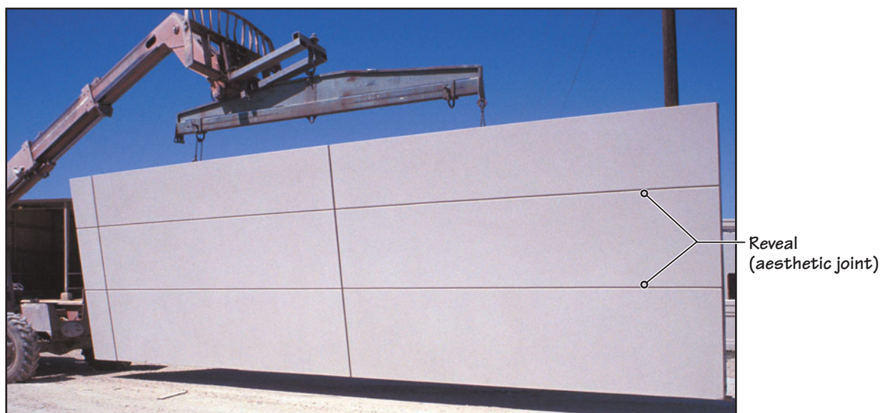
FIGURE 28.51 (a) The front face of a large GFRC panel after light abrasive blasting. It is being lifted for storage in the fabricator's shed.
