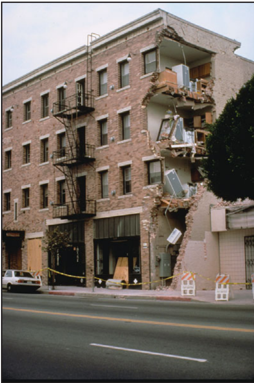
FIGURE 3.23 Damage to an unreinforced masonry building in Santa Monica from the Northridge (California) earthquake on January 17, 1994. (Photo obtained from the World Wide Web using the following URL: http://www.ngdc.noaa.gov/hazard/img/200res/19/19398.tif )
