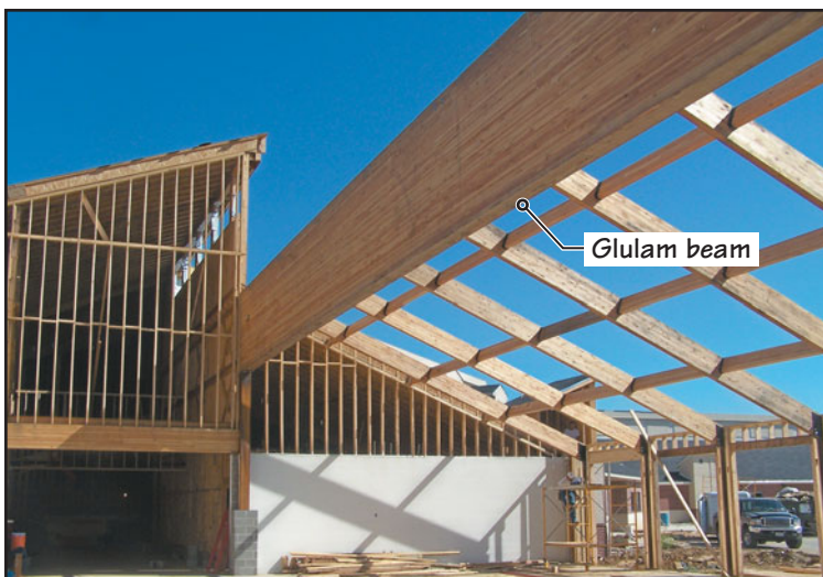
FIGURE 14.2 A 12-in.-wide, 7-ft-deep glulam beam over a long span (82 ft) in Gunter Primary School, Gunter, Texas. Architect: SAI Architects, Keller, Texas. (Photo courtesy of APA—The Engineered Wood Association)
