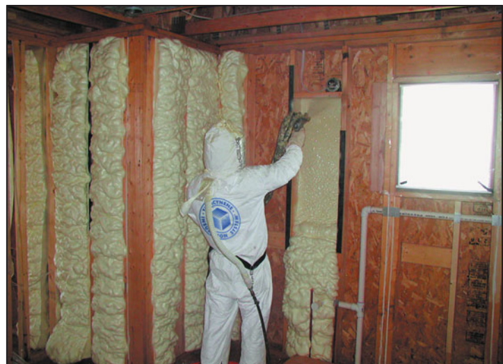
FIGURE 14 Spraying of polyicynene insulation in stud cavities. The insulation expands and cures (hardens) quickly when it is shaved flush with the studs. (Photo courtesy of Icynene, Inc.)
