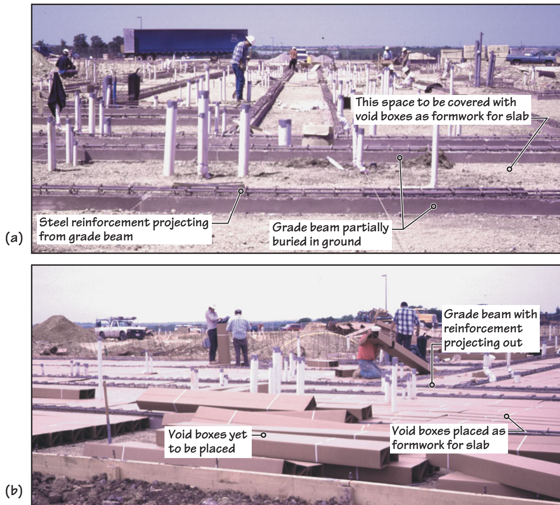
FIGURE 12.36 Construction of the foundation system shown in Figure 12.35. In (a), the grade beams have been partially completed. Figure (b) shows preparation for the construction of the slab-on-ground between the grade beams.
