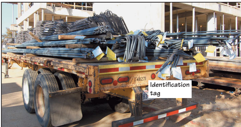
FIGURE 21.39 Bars generally arrive at a construction site bent to shape and cut to required lengths. Tags attached to the bundles identify the building component (beam, column, or slab) to which the bars belong.
