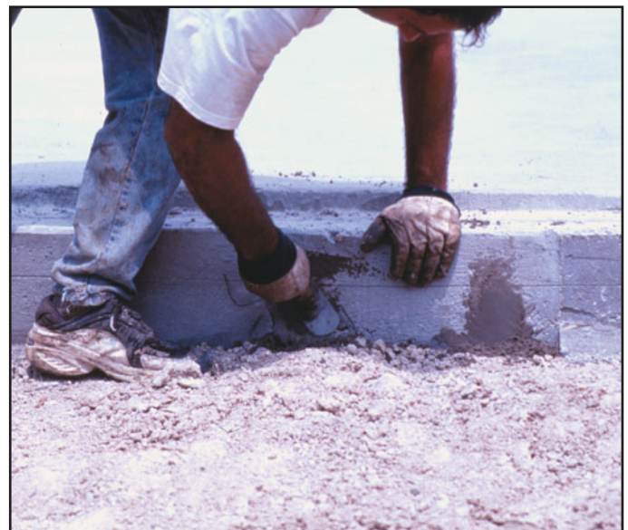
(b) After the tendon is cut, the pocket is filled with a nonshrink grout to prevent corrosion of the tendon.
