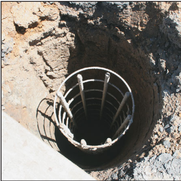
FIGURE 12.14 A pier hole with reinforcement, ready to receive concrete. Steel reinforcing dowels or steel anchor bolts will be placed before concreting; see Figure 12.18. (Photo courtesy of Andrew Kocher)
