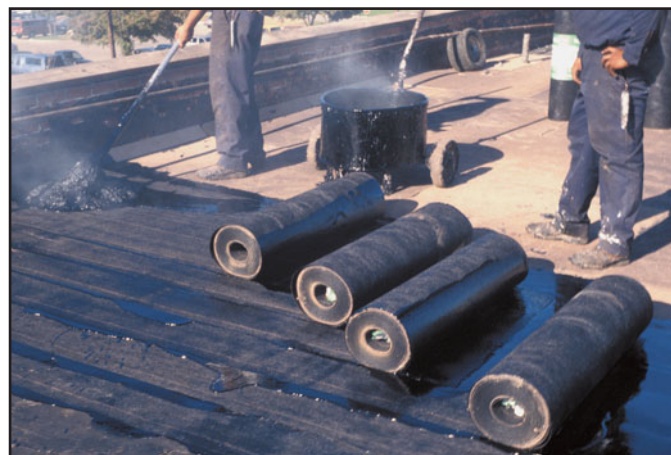
FIGURE 1 Successive built-up roof felts are generally laid in shingle fashion, with the upper felt overlapping the lower felt by a constant dimension. The alternative, applying the felts layer by layer (i.e., in a phased manner), has several disadvantages, and is not used.
