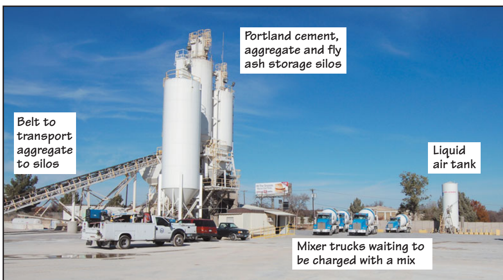
FIGURE 21.20 An overview of a ready-mix concrete plant. Liquid air may be needed in the concrete mix in warm weather to control its temperature. Ice may be used as an alternative, depending on availability and cost.
