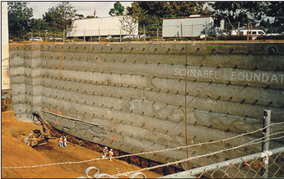
FIGURE 11.27 View of a soil-nailed excavation support. (Photo courtesy of Schnabel Foundation Company)
