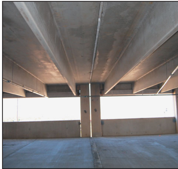
FIGURE 9.5 Building separation joint with two columns in a reinforced concrete building. Because the building is under construction, daylight is showing through the joint between the columns. In a completed building, the joint is sealed and covered with a joint cover, as is the case here for the separation joint in the floor.
