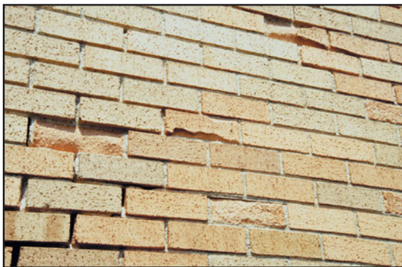
FIGURE 24.9 Spalling of bricks due to freeze-thaw action. In freeze-thaw action, the water absorbed by a wall expands on freezing, producing compressive stresses in the wall. Over repeated freeze-thaw cycles, a wall (made of a low-strength material) spalls, that is, crumbles and falls off.
