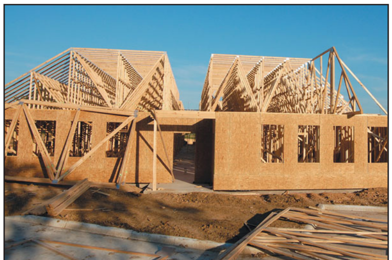
FIGURE 15.35 Prefabricated wood trusses are commonly used in buildings where roof spans are large. Prefabrication reduces on-site labor and hence makes trusses a popular alternative in regions with unfavorable weather conditions or high labor costs.
