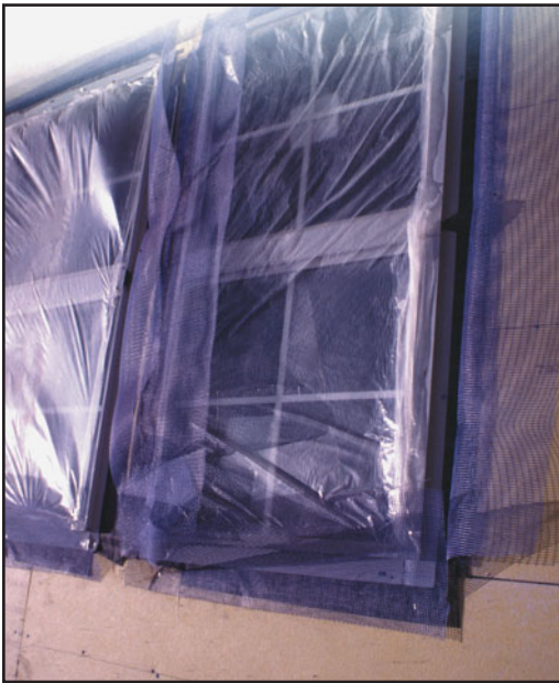
FIGURE 31.8 Aluminum windows were installed in this high-rise condominium building before the exterior (EIFS) wall finish was applied. The windows were, therefore, protected from damage, as shown here.
