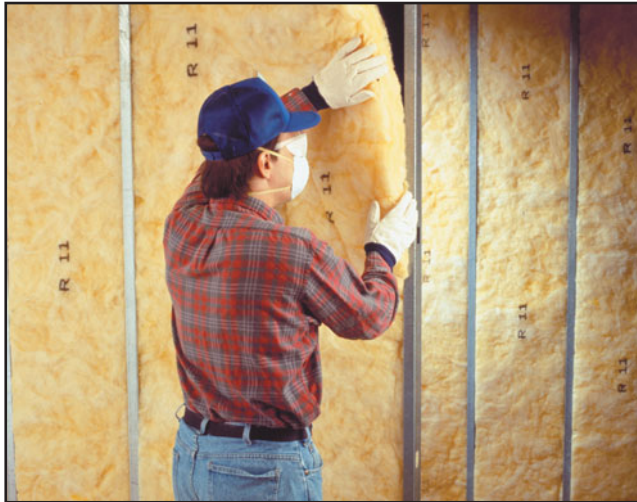
FIGURE 2(a) Unfaced fiberglass insulation installed between studs. The insulation will be covered with a vapor retarder (see Figure 4) before gypsum board is installed on the studs. (Photo courtesy of CertainTeed Corporation)
