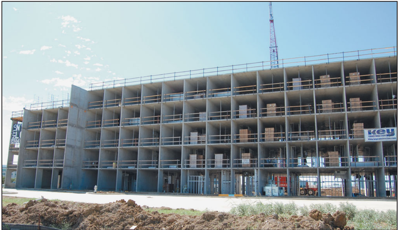
FIGURE 26.26 A five-story hotel building under construction. The structure of the building comprises sitecast reinforced-concrete bearing walls, constructed using steel tunnel forms. The walls and floor slabs of this building are 5 in. thick.
