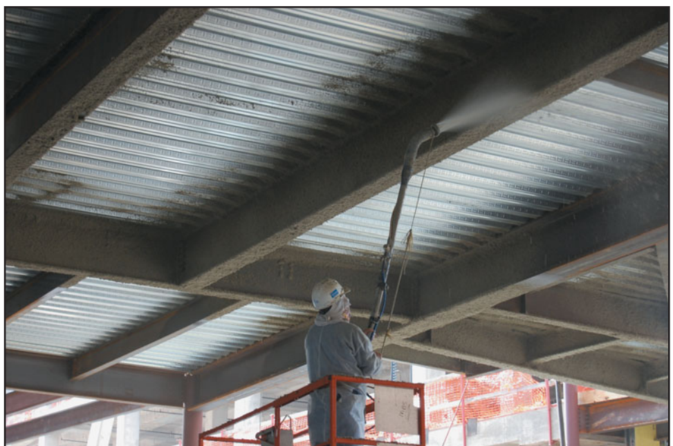
FIGURE 18.35 Spray-on fire protection of a steel floor assembly. Observe that only the floor beams are protected. Fire protection is generally not necessary for the floor deck because of the concrete topping.
