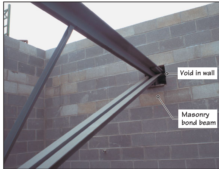
FIGURE 26.11 (b) Support for joists of the building in Figure 26.11(a). Voids, which contain steel bearing plates, are left in the wall at support locations during the construction of the wall. A continuous masonry bond beam is provided under the voids.
