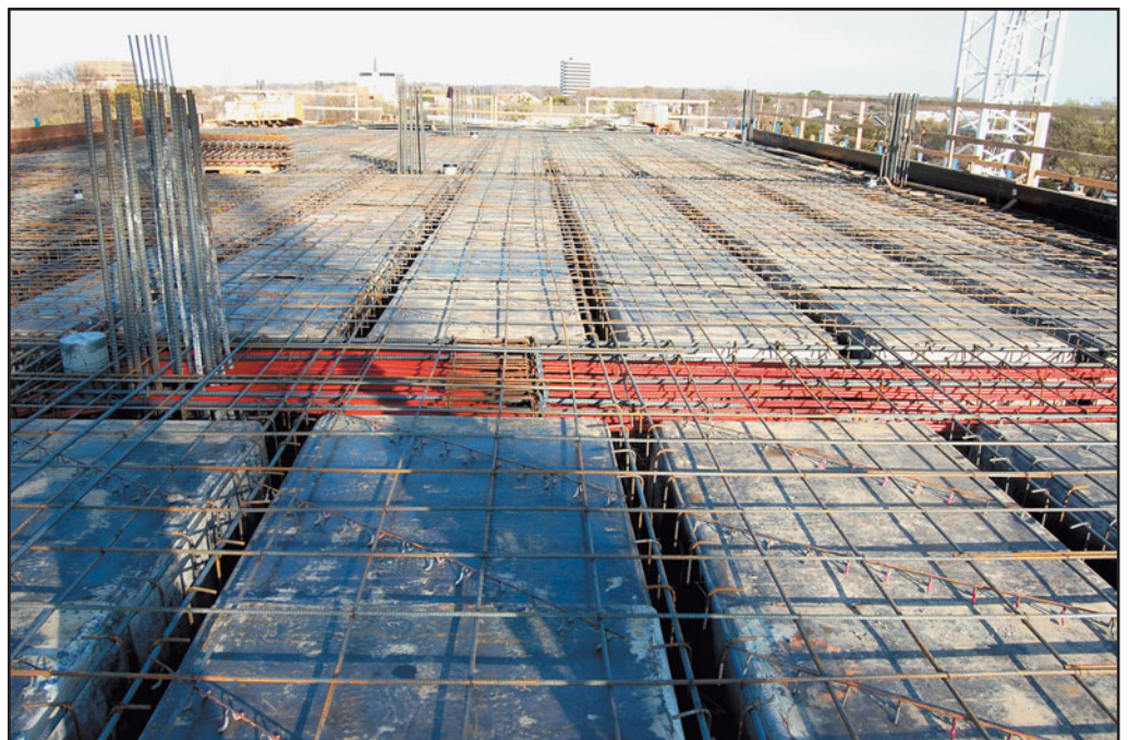
FIGURE 23.21 A wide-module, one-way joist floor with posttensioned (PT) supporting beams. Note the use of (conventional) reinforcement in the slabs and joists. The beams have both conventional reinforcement and posttensioning tendons (red color). PT beams are commonly used in a one-way joist floor to reduce beam size so that joists and beams have the same depth.
