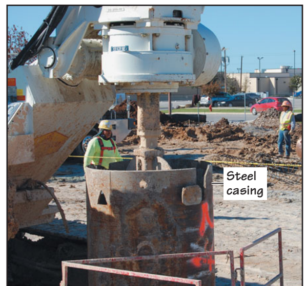
FIGURE 12.17 Steel casing being rotated to push it into hard soil (or rock) to seal its bottom against the entry of water.
