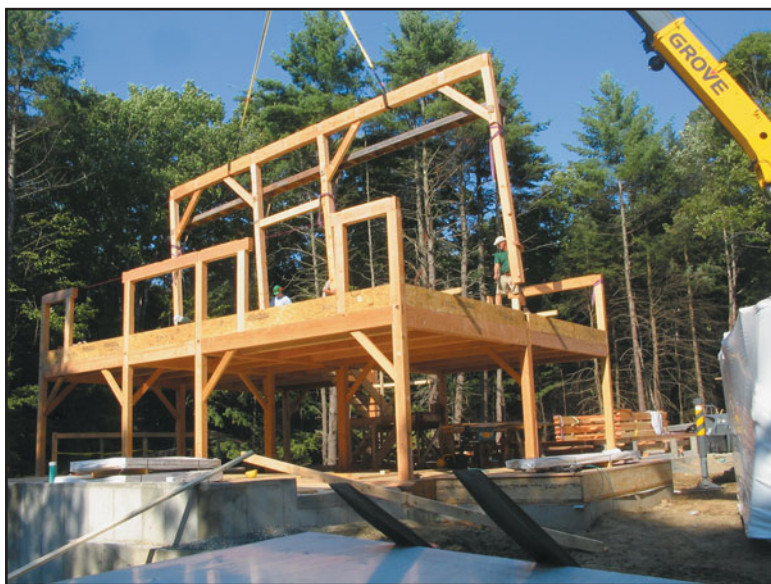
FIGURE 11 A timber frame residence under construction showing a pre-fabricated bent (frame) being installed. (Photo courtesy of Bensonwood Inc.)
