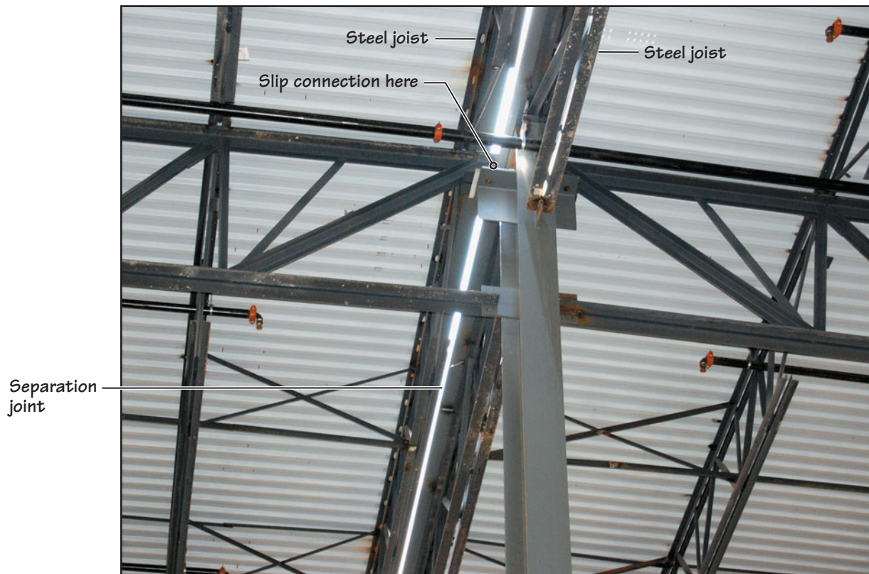
FIGURE 9.8 Building separation joint in a steel frame building using a single column. Because the building is under construction, daylight is showing through the separation joint. In a completed building, the joint is sealed and covered with a joint cover (see Chapter 19 for details of the separation joint). Observe the provision of a steel joist on each side of the separation joint.
