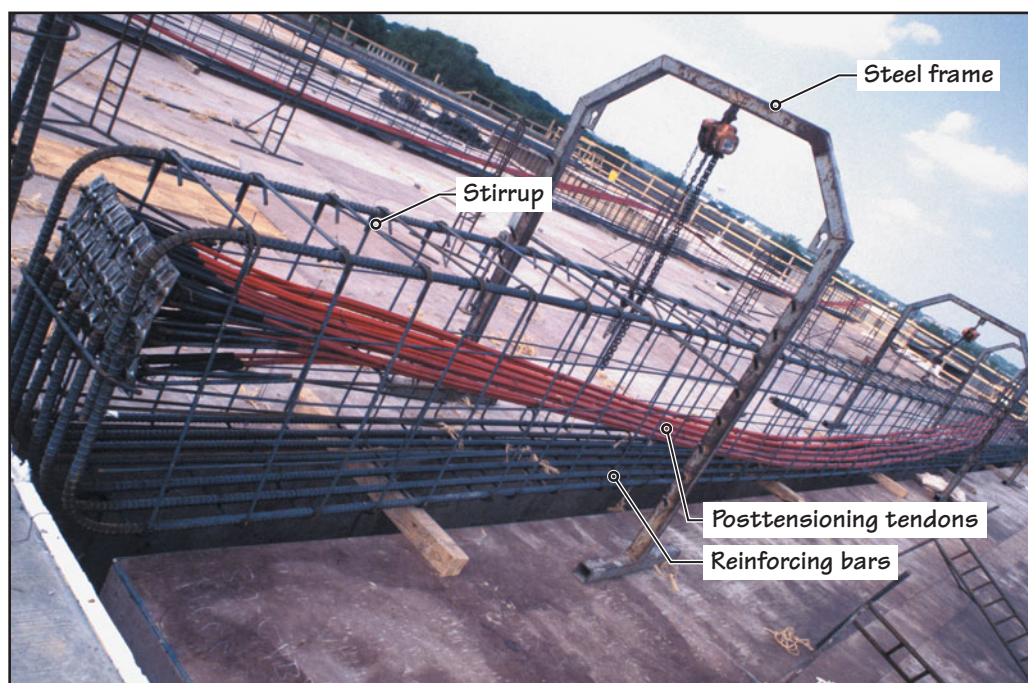
FIGURE 23.19 A cage for a concrete beam consisting of conventional reinforcement and posttensioning tendons (red color) ready to be lowered into the beam form. Observe the drape (generally parabolic) provided in posttensioning tendons to balance the stresses created by gravity loads on the beam. The steel frames shown are used to make the cage. They will be removed after the cage has been placed in the form. Reinforcement for the slab is yet to be completed. Figure 23.20 shows the same beam after its reinforcement has been lowered and the reinforcement and posttensioning tendons for the slab are in place.
