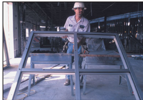
(c) The two windows have become one window with a common mullion without the use of fasteners.
