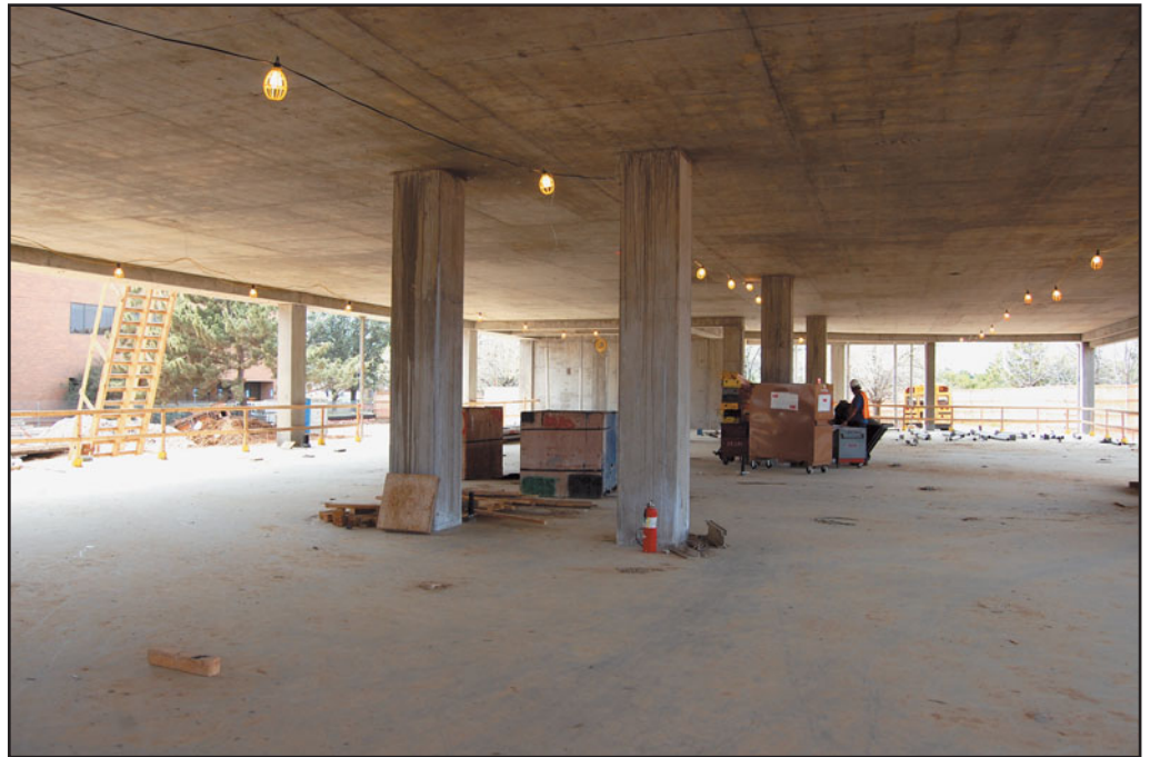
FIGURE 23.16 A flat-plate slab in an office building under construction. Observe the use of perimeter beams, which may be required with heavy exterior wall cladding. Flat-plate slabs without perimeter beams are common. Columns may be rectangular, square, or round.
