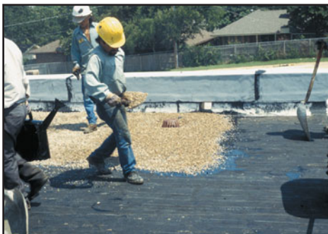
FIGURE 33.3(e) The bitumen flood coat is covered with stone aggregate. For a small roof, shovels are used to spread the aggregate.
