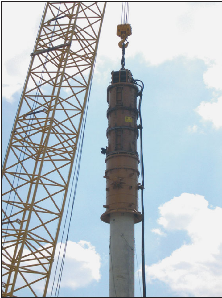
FIGURE 12.8 A round concrete pile being driven by a hydraulic impact hammer. (Photo courtesy of Pile Driving Contractors Association [PDCA], Orange Park, Florida)
