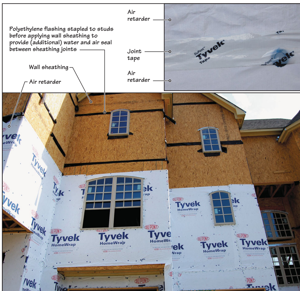
FIGURE 6.5 An air retarder wrapped over the exterior wall sheathing of a three-story wood frame condominium building. The photograph was taken while the installation of the air retarder was in progress. After installation of the air retarder over all of the exterior sheathing is completed, exterior cladding will be installed. The magnified part of the air retarder shows the self-adhering tape between the air retarder joints.
