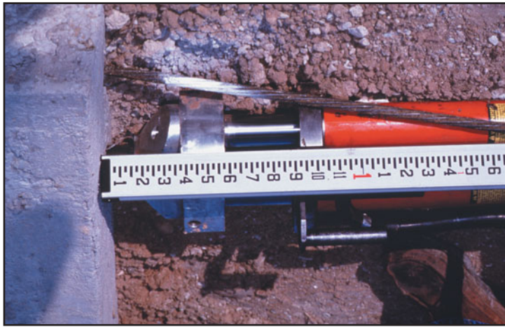
(a) A tendon being stressed by the jack. The amount of prestressing force in the tendon is indicated by the gauge reading and verified by a predetermined elongation of the tendon.
