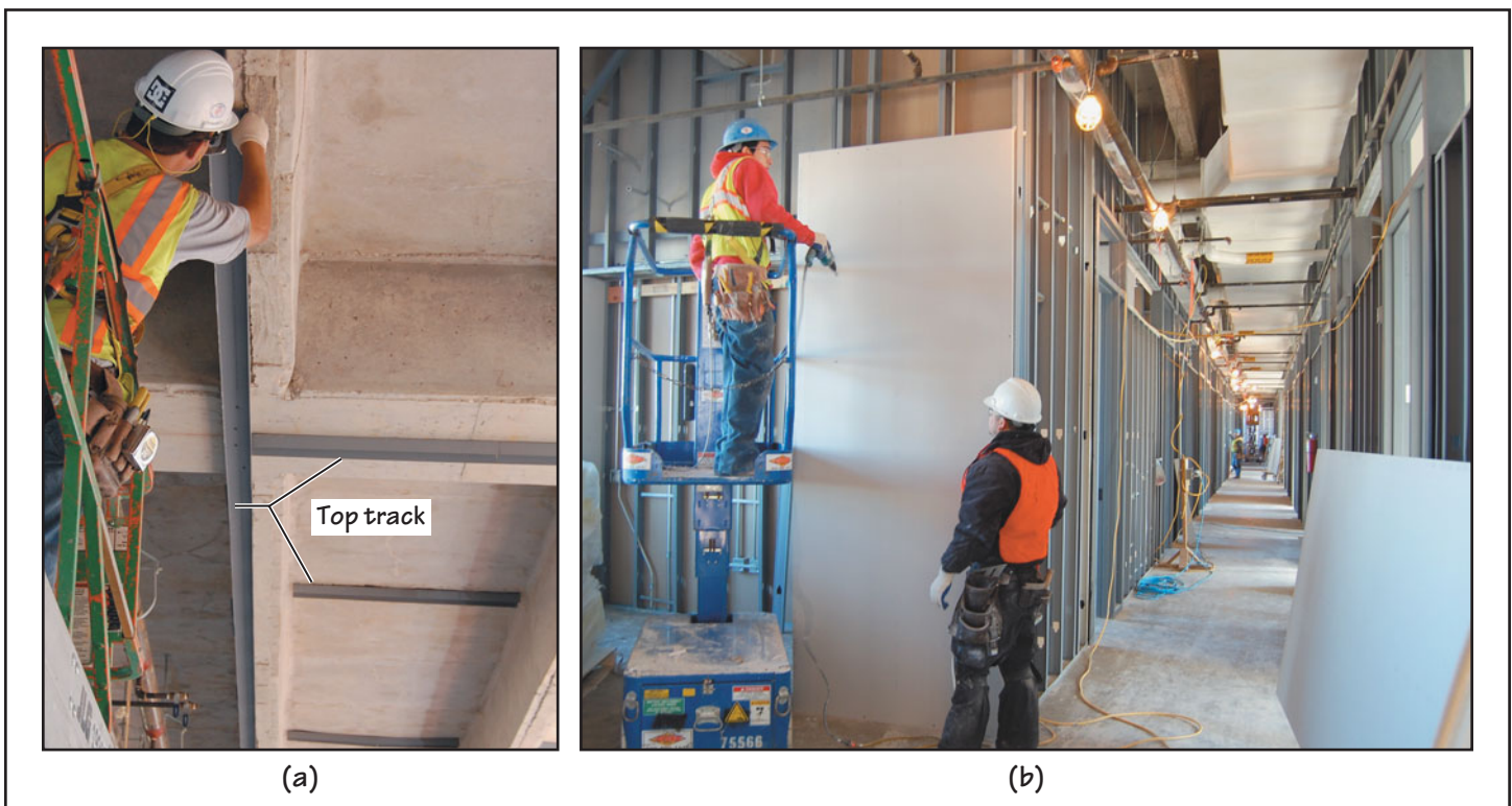
FIGURE 20.8 (a) A worker fastens the top track for an interior partition to the underside of the floor slab. (b) Gypsum board being fastened to CFS framing of an interior partition.
