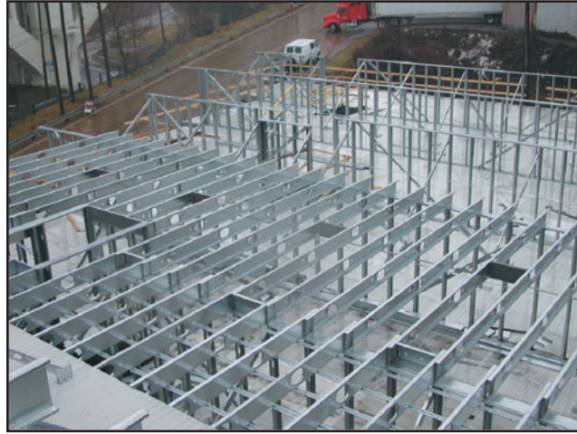
FIGURE 20.22 Layout of floor joists in a typical CFS structure. (Photo courtesy of Dietrich Metal Framing)
