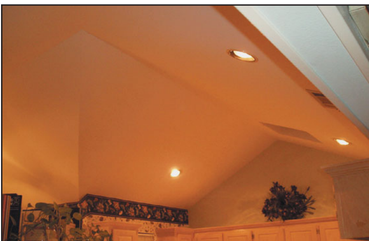
FIGURE 37.4 A typical gypsum board ceiling attached to the wood framing in a residential application.
