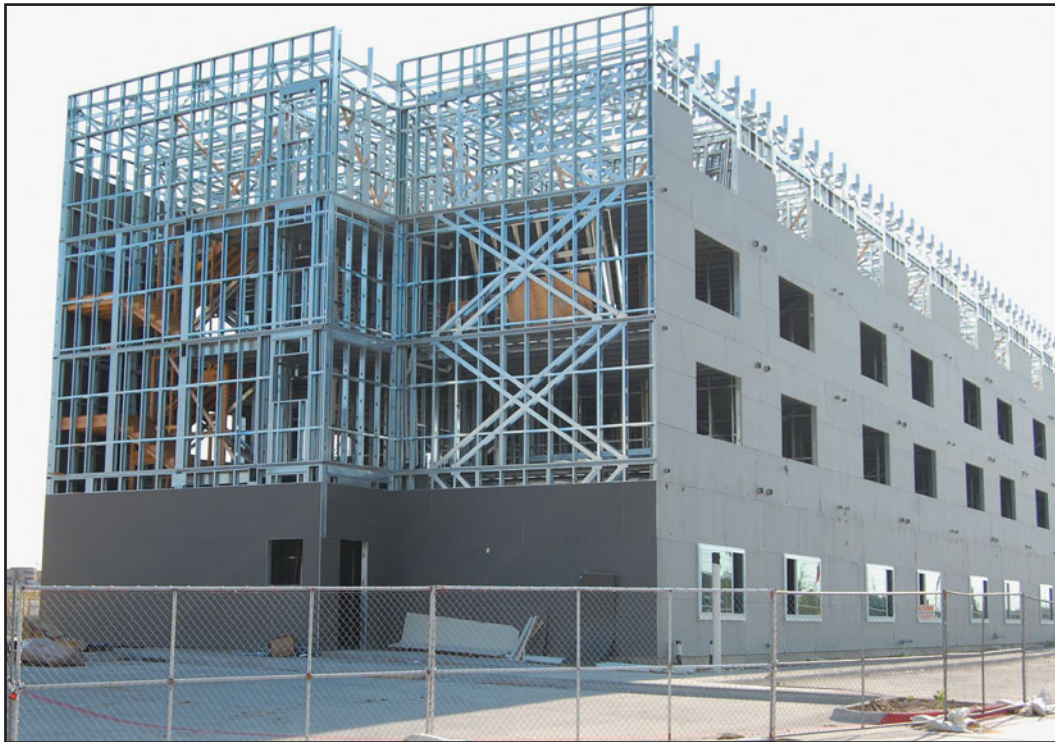
FIGURE 20.12 CFS framing for a six-story load-bearing wall hotel building in progress. In this building, all assemblies (walls, floors, and roof) are framed with CFS members.
