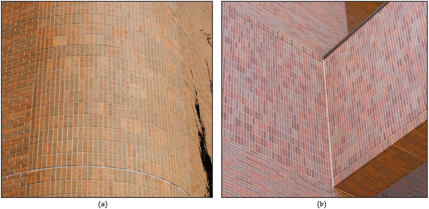
FIGURE 24.22 A stack-bonded brick wall used (a) to achieve a sharp curve and (b) for aesthetic reasons.
