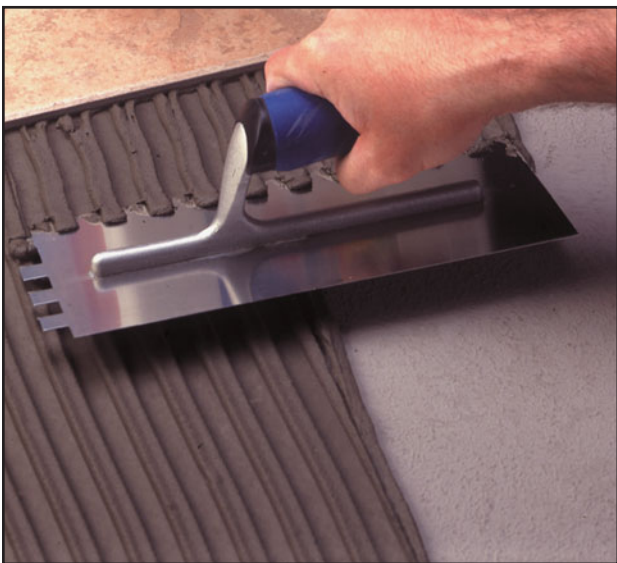
FIGURE 36.5 A closer view of mortar being spread using a notched trowel (in this case, an epoxy mortar). (Photo courtesy of Mapei Corp.)
