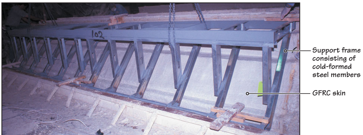
FIGURE 28.56 After spraying and consolidating the mix for the GFRc skin on the mold, a cold-formed steel supporting frame is placed against the mold and bonding pads are formed.
