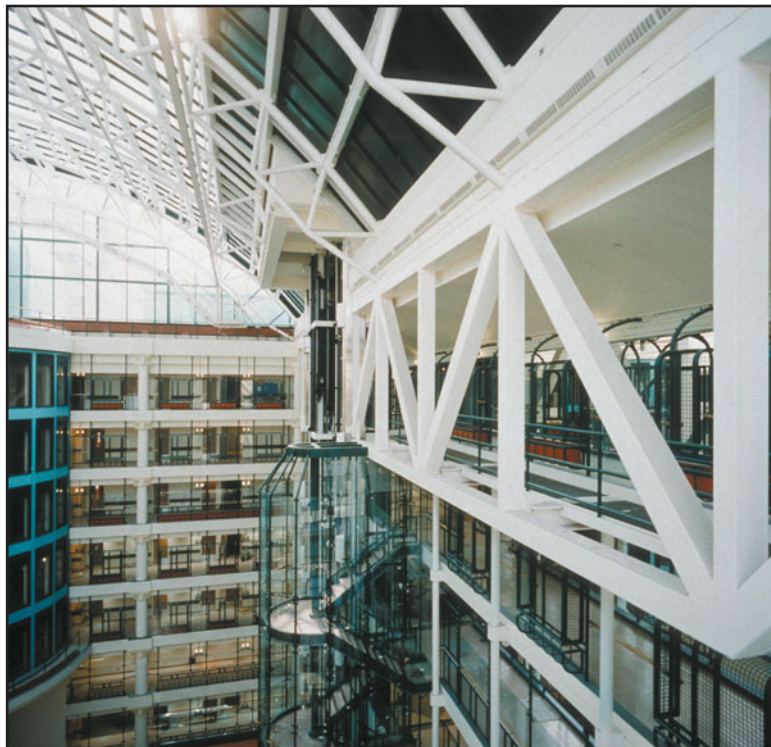
FIGURE 18.36 A steel truss painted with intumescent paint providing a 1-h fire rating, Hospital for Sick Children, Toronto, Ontario. (Photo courtesy of AD Fire Protection Systems, Scarborough, Ontario. Architect: Zeidler Roberts Partnership. Photo by Lenscape Inc.)
