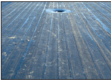
FIGURE 33.3(c) This image shows the roof after all built-up felt plies have been applied. The roof is now ready to receive the flood coat of bitumen and the stone aggregate surfacing, as shown in the following two images.
