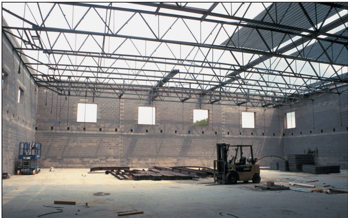
FIGURE 26.11 (a) A gymnasium with 12-in.-thick CMU bearing walls (in a box-type floor plan) and a steel joist roof. The joists span nearly 100 ft between walls and are approximately 60 in. deep.
