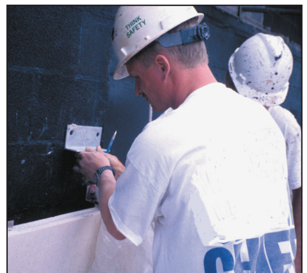
FIGURE 29.32 Anchorage of a J-shaped shelf angle clip to a CMU backup wall whose surface has been treated with a liquid-applied air-weather retarder.
