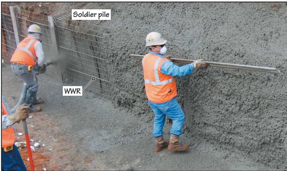
(a) Shotcreting over WWR and finishing of an already shotcreted part of a wall
