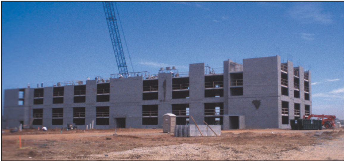
FIGURE 26.23 (a) This and the following five images show the construction of an eight-story load-bearing masonry hotel building. The building, with a cross-bearing wall plan (see Figure 26.14), is in its early stages of construction.
