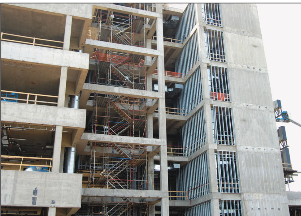
FIGURE 7.12 A cast-in-place reinforced concrete building (under construction). It is not possible to precisely judge its type of construction [Type I(A), Type I(B) or Type II(A)] without examining the construction drawings of the building because the fire rating of a cast-in-place reinforced concrete building is a function of the dimensions of the structural members and the concrete cover over steel reinforcement. However, such a building is likely to be a Type I(A) or Type I(B) construction, probably Type I(A).
