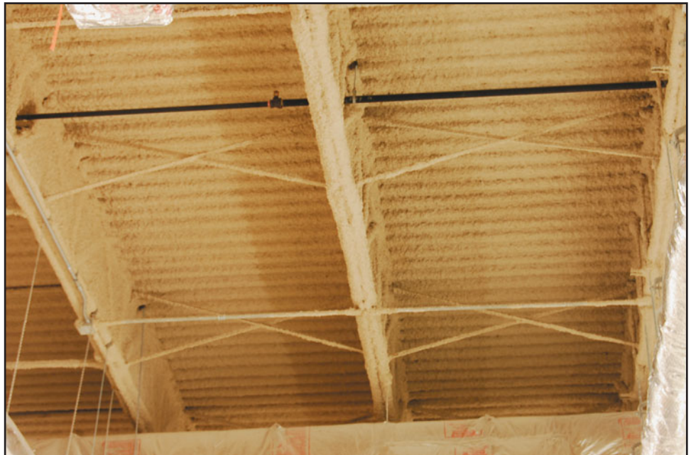
FIGURE 18.34 Spray-on fire protection of a steel roof assembly. Observe that both joists as well as the roof deck are protected.
