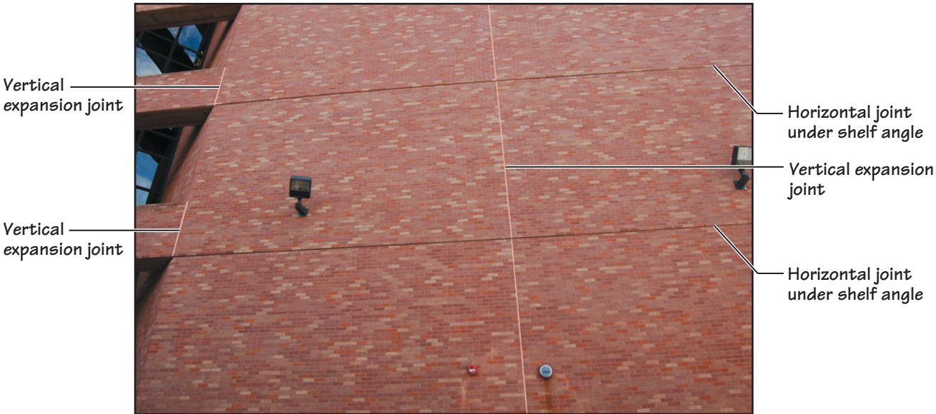
FIGURE 28.15 Continuous vertical expansion joints in brick veneer. Also note the continuous horizontal joints under the shelf angles.
