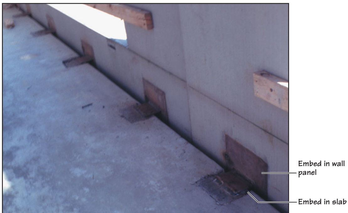
FIGURE 26.38 Details of the connection between tilt-up wall panels and the elevated ground-floor slab (with an underlying crawl space).
