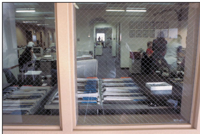
FIGURE 30.27 Wired glass in a fire-rated window between a parking garage and an office room.
