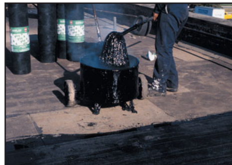
FIGURE 33.3(a) With a bucket full of hot bitumen and a mop, a roofer begins to lay a built-up roof.
