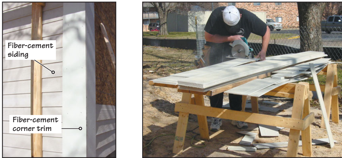
FIGURE 16.10 (a) Manufacturers of fiber-cement sidings provide trim materials to match their sidings. (b) Site cutting of fiber-cement siding.
