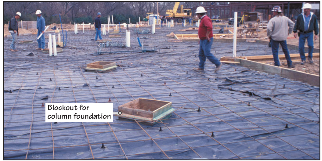
FIGURE 22.37 An isolated slab being inspected before concreting. Observe the vapor retarder and the reinforcing bars supported on chairs. Also observe the blockouts for columns, which isolate the slab from the building's structure.
