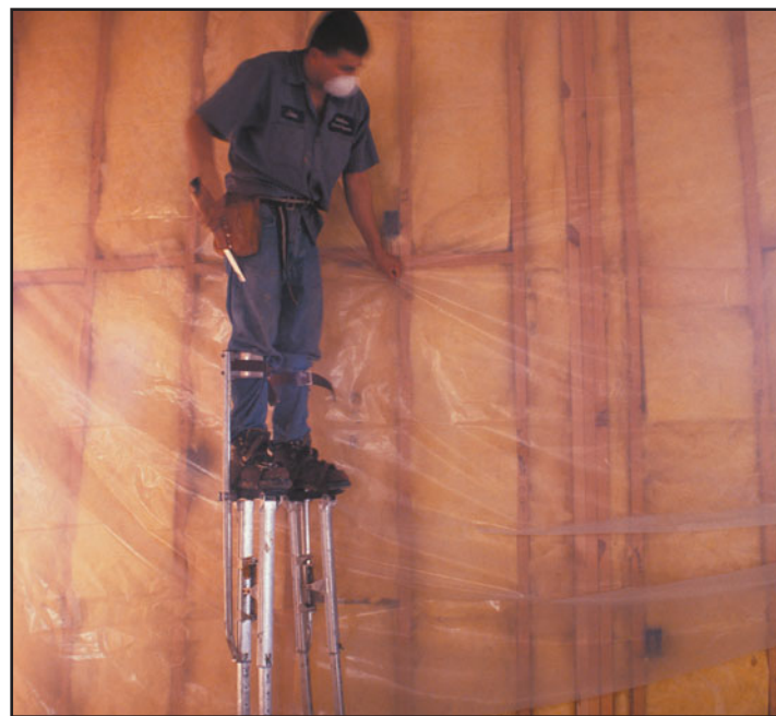
FIGURE 4 A clear polyethylene sheet vapor retarder being installed over unfaced fiberglass insulation between wood studs.
