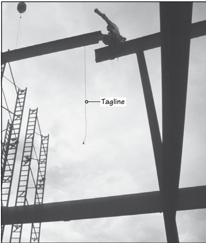
FIGURE 19.20 A steel erector (with his body harness tied to the beam on which he sits) maneuvers the new beam into position, initially using the rope attached at the end of the beam and later by hand. The rope is referred to as a tagline in erection vernacular.
