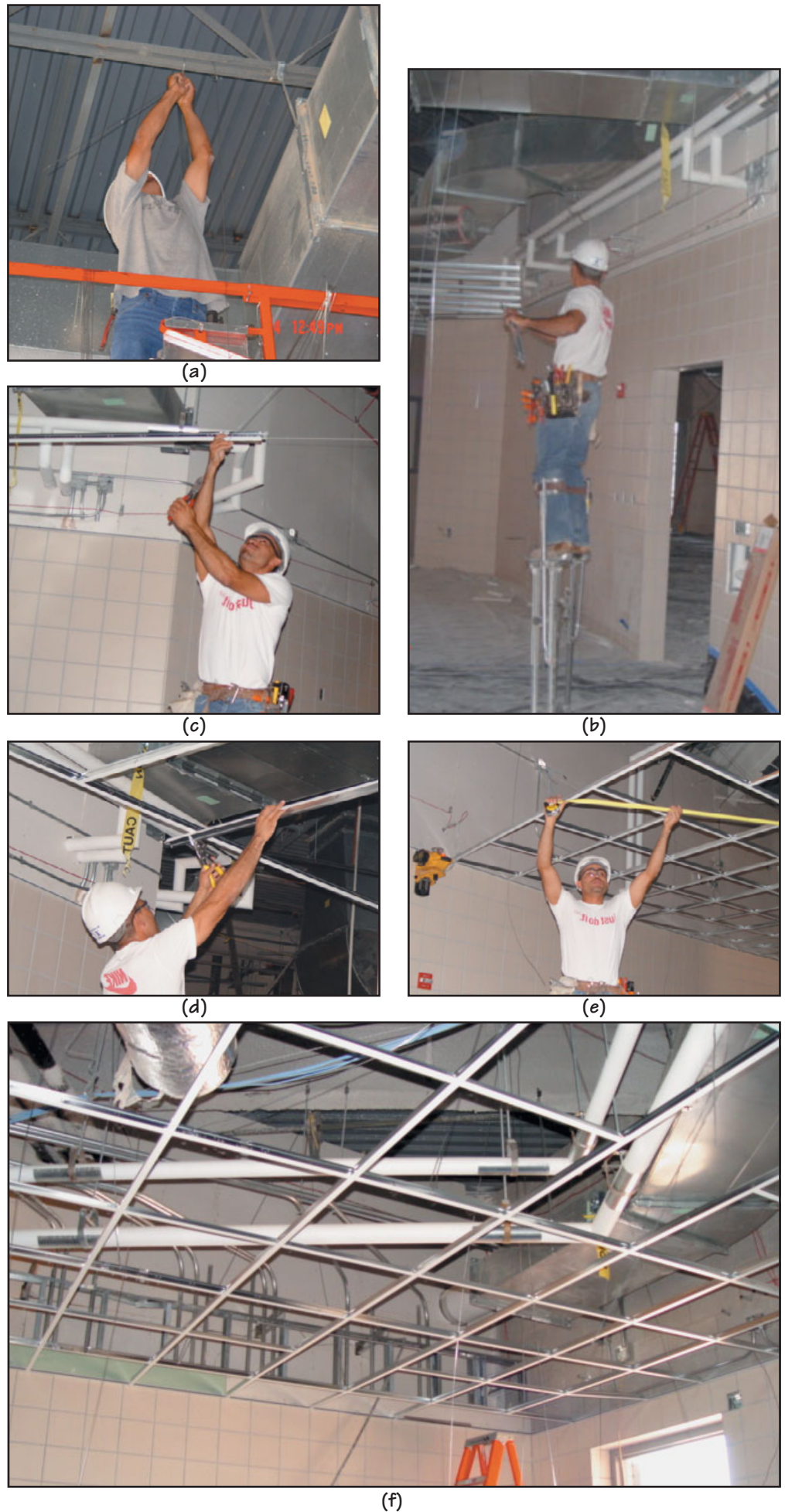
FIGURE 37.8 Installation of a suspended grid. (Photos of Vaden's Acoustical & Drywall, Inc. by Gary Yancy of USG Building Systems). (a) Attaching steel hanger wire to the steel structural joist above. In this case, the hanger wire is tied to the steel joist. When a concrete slab or metal deck is present, a hanger wire, with an integral clip angle, is usually powder-fastener attached. Hanger wires are always attached to the building structure, not to building utilities. (b) Layout begins by establishing the location of the main runners. For most ceilings, installers will use stilts to assist in installation or will use a rolling scaffold. (c) Using string and a laser level (see (e) ), installers establish main runner locations. (d) Until permanent attachments can be made, installers clamp intersecting tees together. (e) Continuing with installation; notice the laser level at the wall. (f) Final suspended grid installation, including openings for light fixtures.
