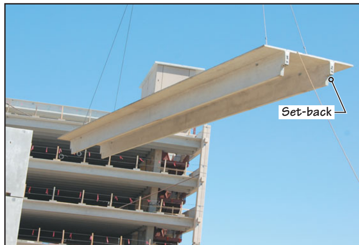
FIGURE 23.26 A double-tee floor unit being flown into position in the total precast building in Figure 23.25. The setbacks in double-tee stems reduces floor height.
