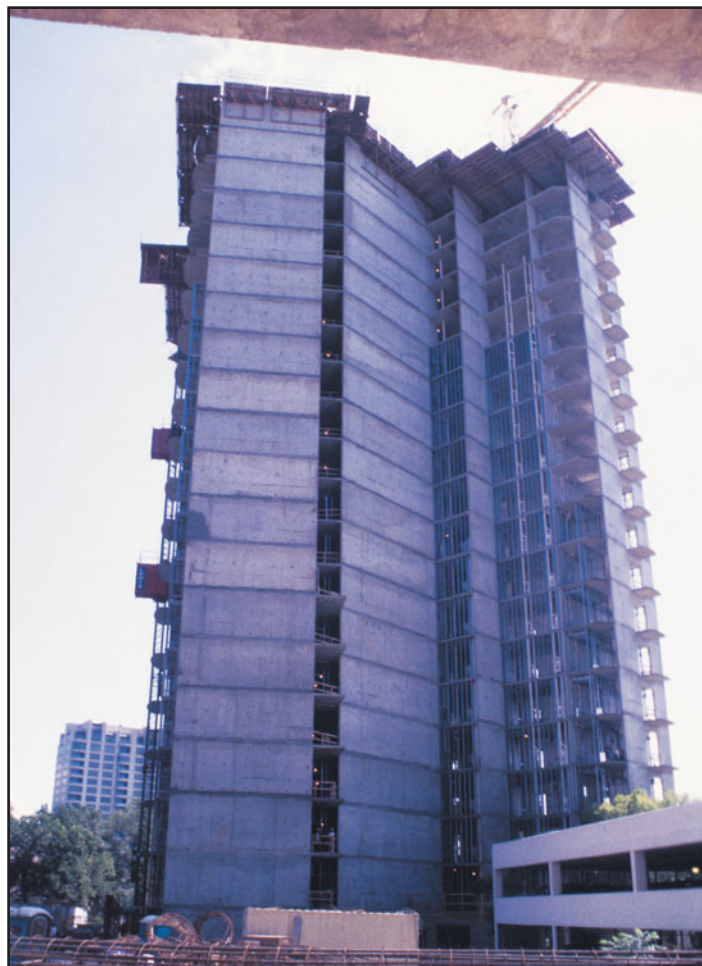
FIGURE 26.27 A 22-story apartment building under construction. The structure of the building comprises sitecast reinforced-concrete bearing walls, constructed using steel tunnel forms. The walls and floor slabs of this building are 6 in. thick.
