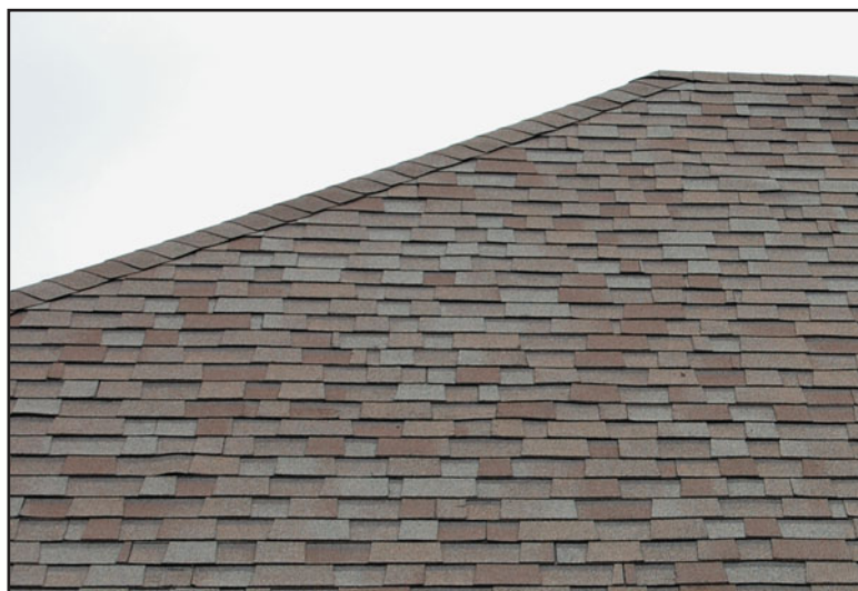
FIGURE 34.21 An asphalt shingle roof showing hip cap shingles and ridge cap shingles. Note that the two types of shingles are identical.
