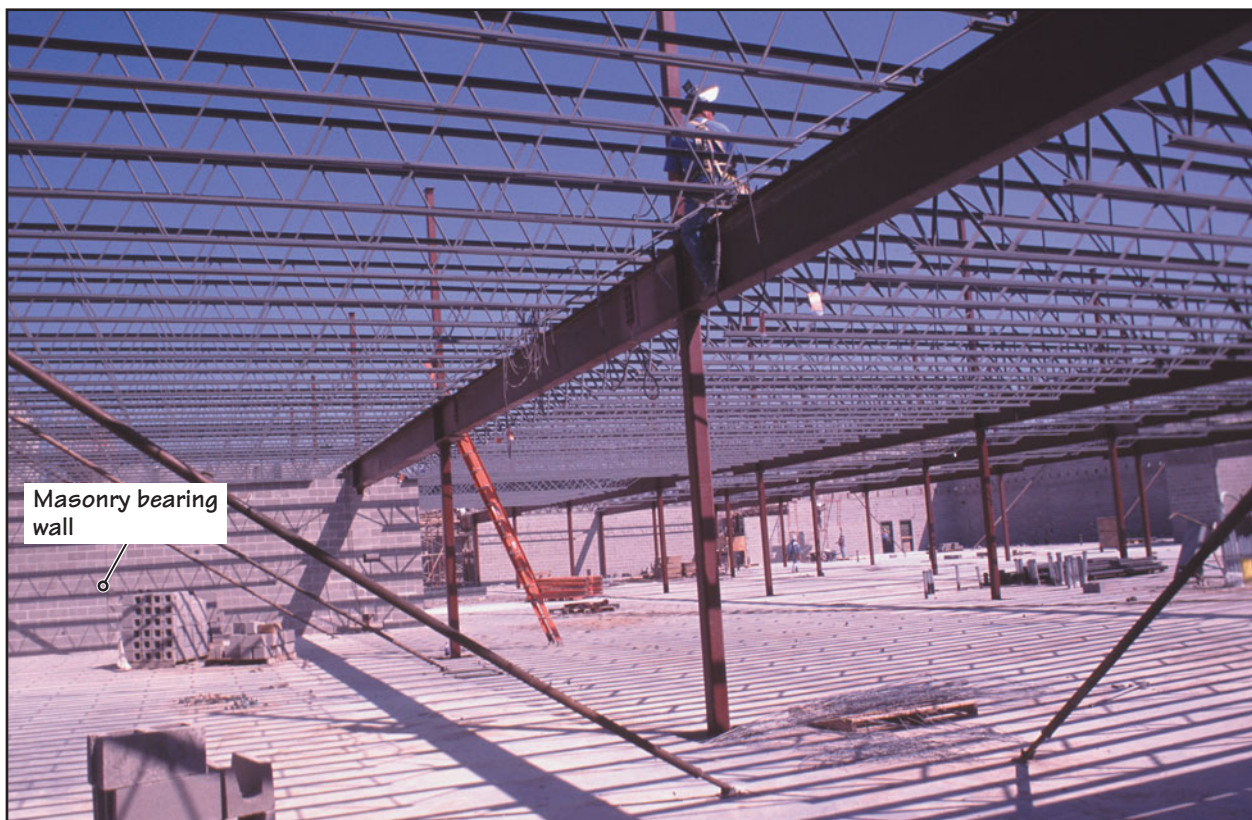
FIGURE 26.24 A school building with exterior load-bearing masonry walls and interior steel frame under construction.
