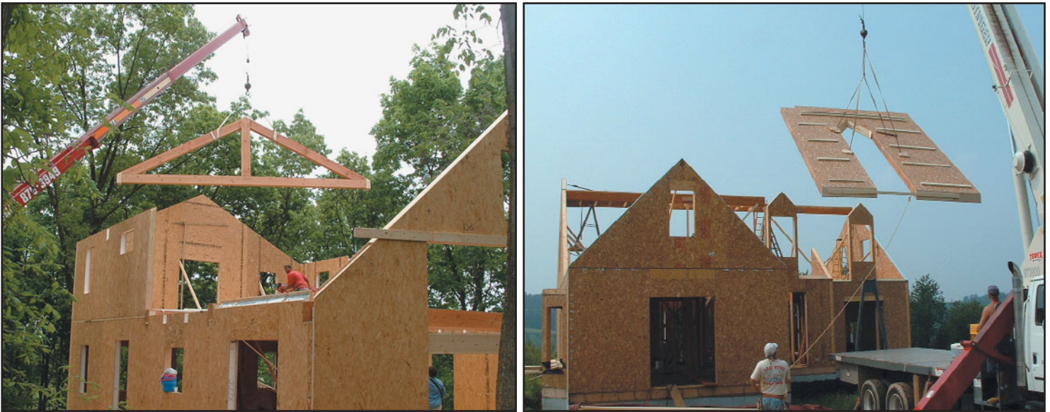
FIGURE 17.1 Two examples of typical structural insulated panel buildings under construction. (Photos courtesy of the Structural Insulated Panel Association [SIPA])
