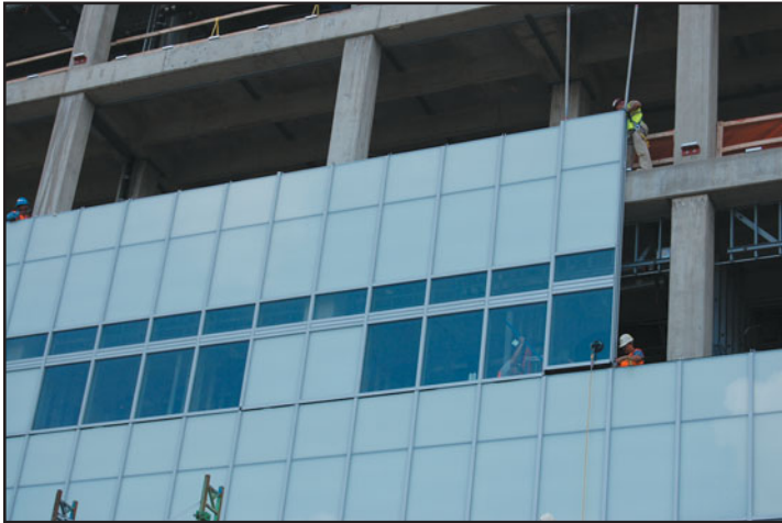
(b) The new unit is installed by placing both of its mullions over the (projecting) splices in the lower unit. The splices function as expansion splices (see Figure 32.3) and also provide lateral-load support to the unit. The lower unit is anchored to the floor structure through a dead-load support to the unit.
