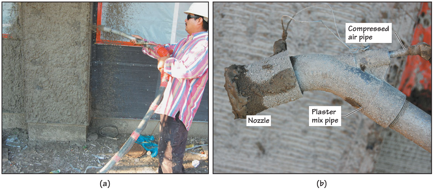
FIGURE 29.6 (a) Spraying of the stucco base coat over metal lath. (b) The pipe used for spraying the stucco mix terminates in a nozzle. The spray action for the mix is provided by a separate compressed-air pipe that also terminates in the same nozzle as the plaster mix pipe.
