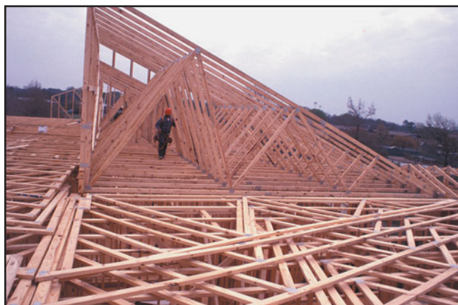
FIGURE 14.18 Mono-slope roof trusses. Two mono-slope trusses laid end-to-end and field connected make a common roof truss. Mono-slope trusses are generally used where a common truss is too large to transport to the site. Wood trusses are generally spaced 24 in. on center.
