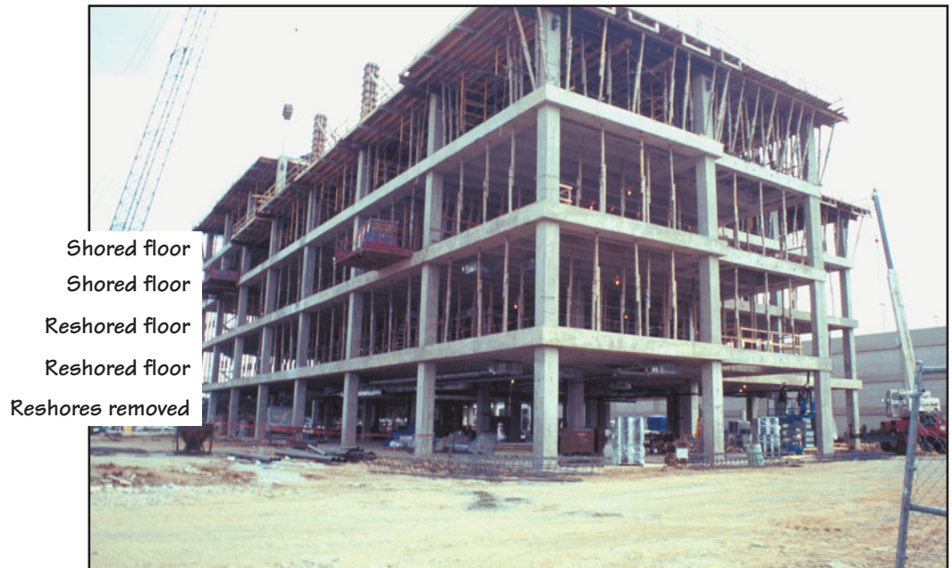
FIGURE 22.12 In this building under construction, the concreting for the top floor has been completed and the forms for the next floor are being installed. The two underlying floors have been reshored, while the reshores from the ground floor have been removed to allow interior construction. As far as possible, reshores must align in the same vertical position from floor to floor.
