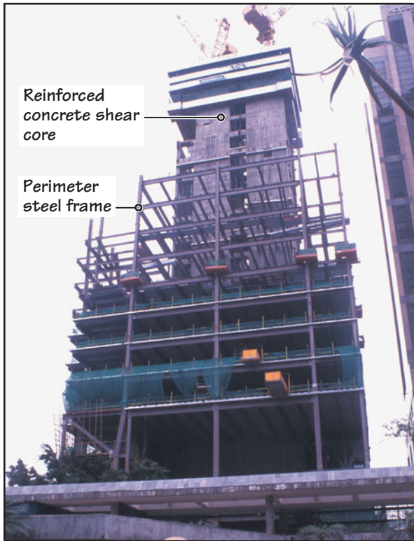
FIGURE 24 A steel-frame building with a reinforced concrete central core under construction in Hong Kong.
