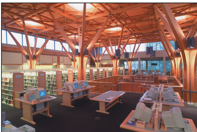
FIGURE 14.3 Glulam columns used in Beaverton Public Library, Beaverton, Oregon. Architect: Thomas Hacker and Associates, Portland, Oregon. (Photo courtesy of APA—The Engineered Wood Association)
