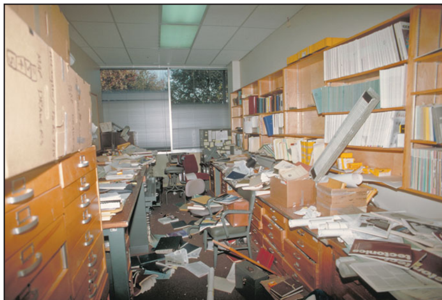
FIGURE 3.24 Effect of earthquake shaking (1989 Loma Prieta earthquake) on the contents of a building's interior. Note that the building envelope is intact. Greater damage could have occurred if the interior fixtures were inadequately anchored. (Photo obtained from the World Wide Web using the following URL: http://pubs.usgs.gov/dds/dds-29/tif/img0040.tif )
