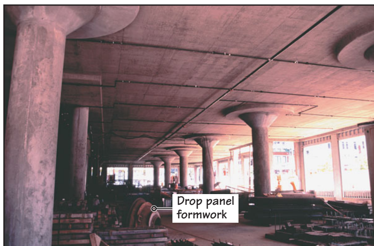
FIGURE 23.18 A flat slab with (round) drop panels and column capitals under construction.
