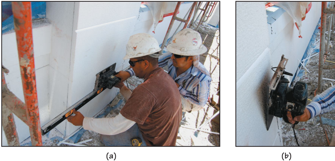
FIGURE 29.24 (a) Cutting of reveals (aesthetic grooves) in the insulation after it has been adhered to the substrate with the help of a groove-making tool and a level. (b) A close-up of the groove-making tool that makes a V-shaped groove. The tool can be adapted to make grooves with different profiles.
