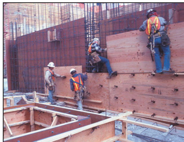
FIGURE 22.32 Workers equipped with safety harness erect the formwork for a reinforced-concrete wall. (See Figure 22.33 for details.)
