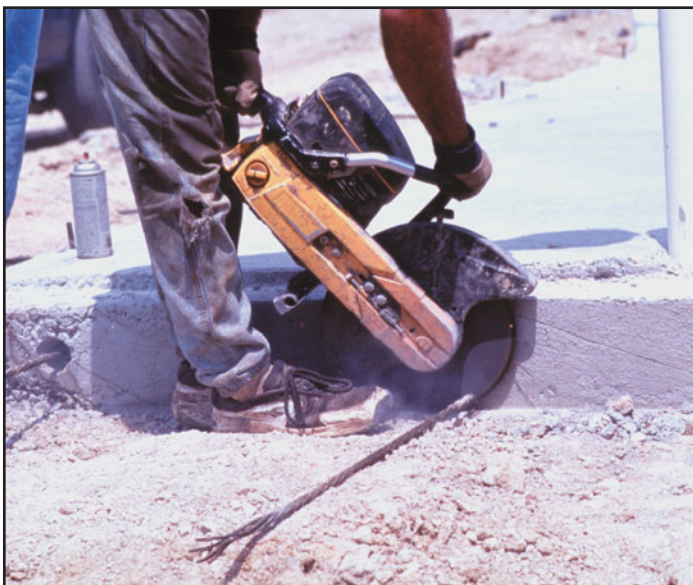
(a) After stressing, the tendon is cut with a saw (or a torch).
