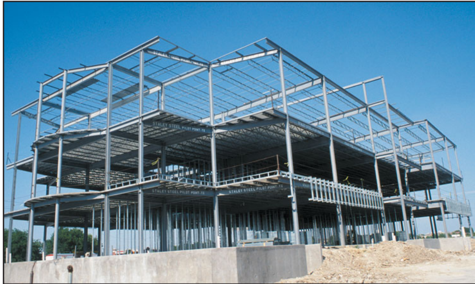
FIGURE 20 A typical steel rigid frame building. Observe the absence of braced bays, which gives greater freedom in organizing the interior spaces and building's facade.
