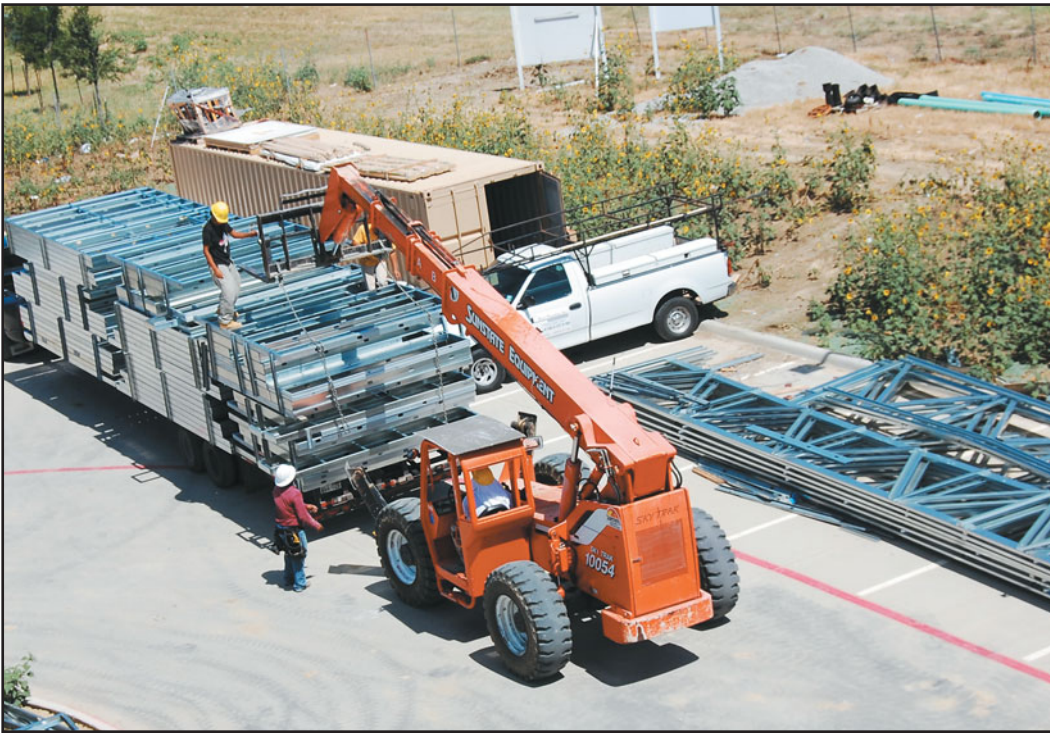
FIGURE 20.16 A forklift is unloading prefabricated CFS assemblies from the truck. CFS wall, floor, and roof assemblies are generally prefabricated off-site into units and brought to the site for installation and connections.
