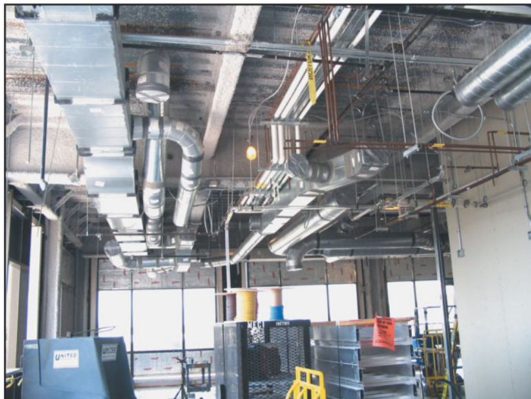
FIGURE 37.2 In most buildings, there are usually many utilities located overhead, as shown in this image. Because many of these utilities require periodic access, an acoustical suspended ceiling is frequently selected. (Photo courtesy of HKS Inc.)
