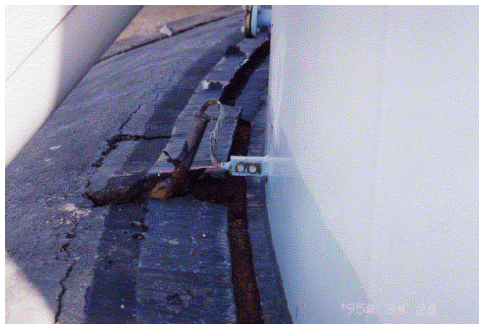
(e) Pulled out of earthing wire
