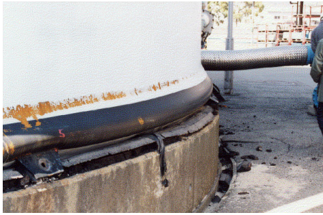
(c) Elephant foot bulge type buckling of tank wall
