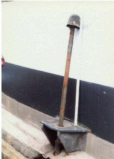
(a) Pulled out of anchor bolt
