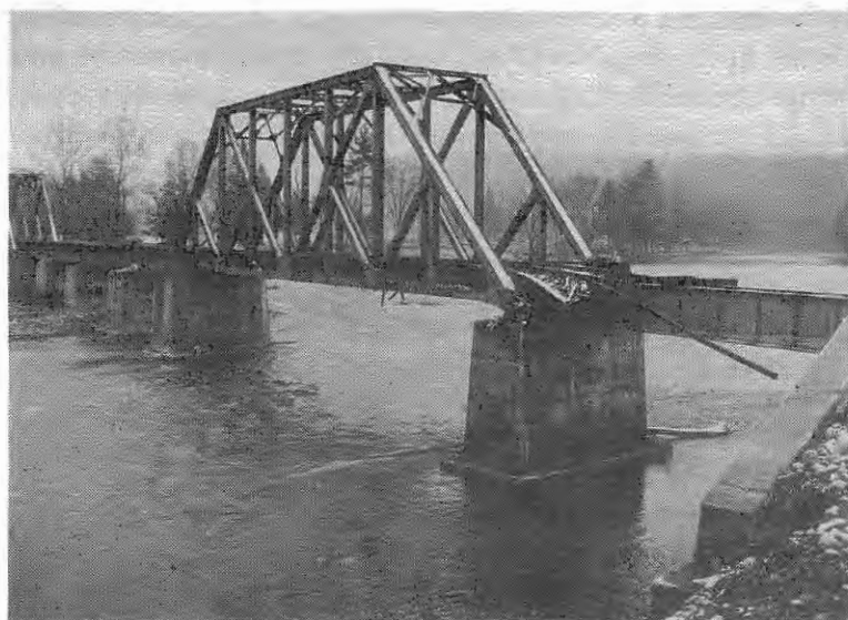
Sample of the results of a $3 trillion deficit in U.S. infrastructure spending: an abandoned railroad bridge in West Virginia.
